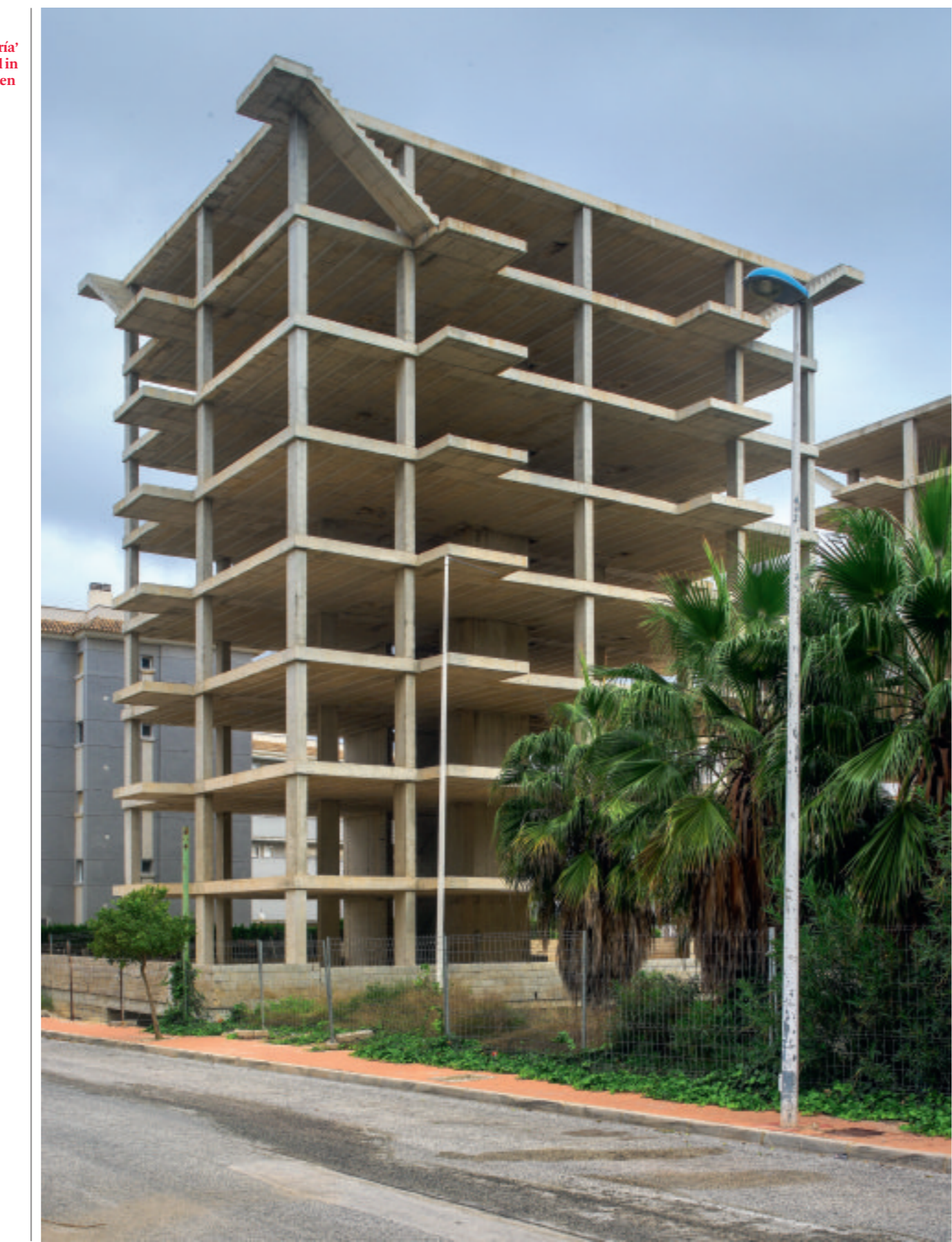
Links: 'Almoradí' (2019), rechts: 'Almería' (2019). Overal in Spanje wachten betonnen skeletten op financiering.
